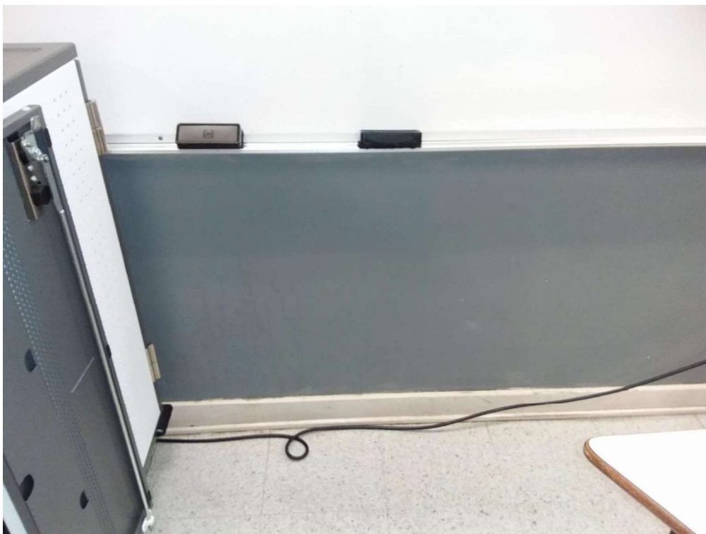
Lead, None (L0008) Wall, Classroom (Location #: 36) Grey
