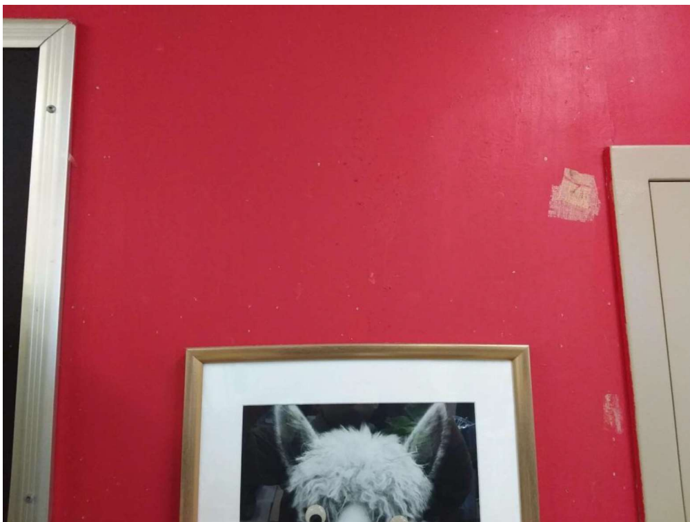
Lead, High (L0010) Wall, Classroom (Location #: 56) Red
