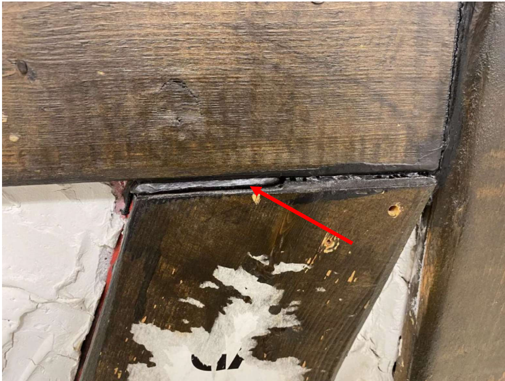
Confirmed Asbestos (S0003A-C), Wall, Interior, Black Caulking, Cafeteria (Location #: 27) On wood seams
