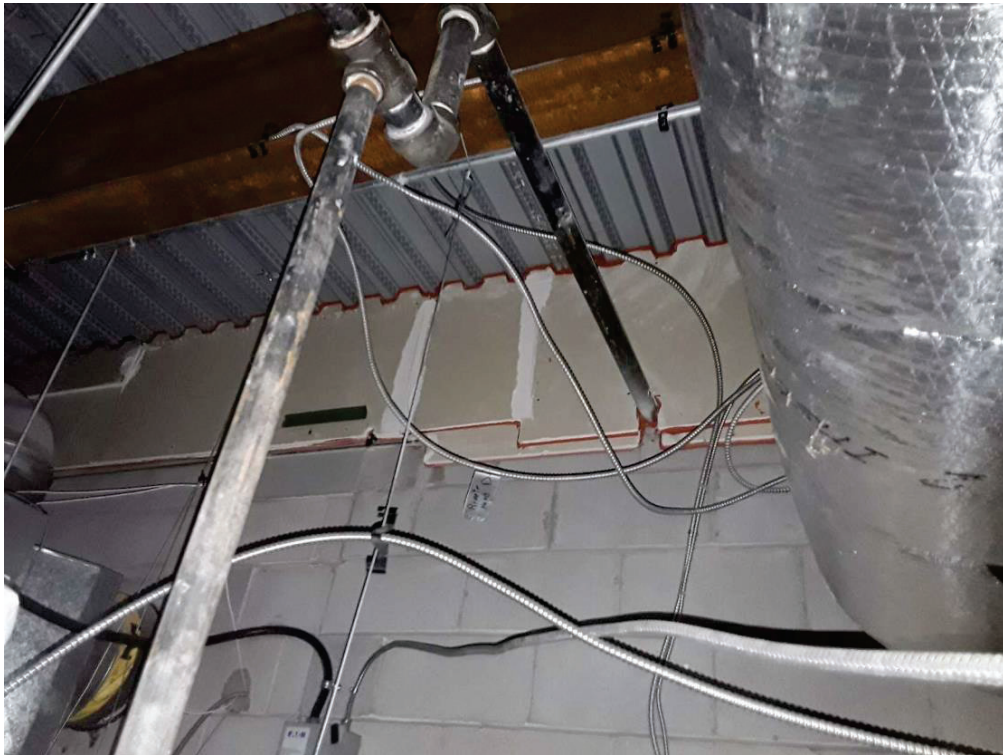
V0002 (None), Red firestopping mastic, Floor 1 Corridor (Location #: 1) Perimeter walls
