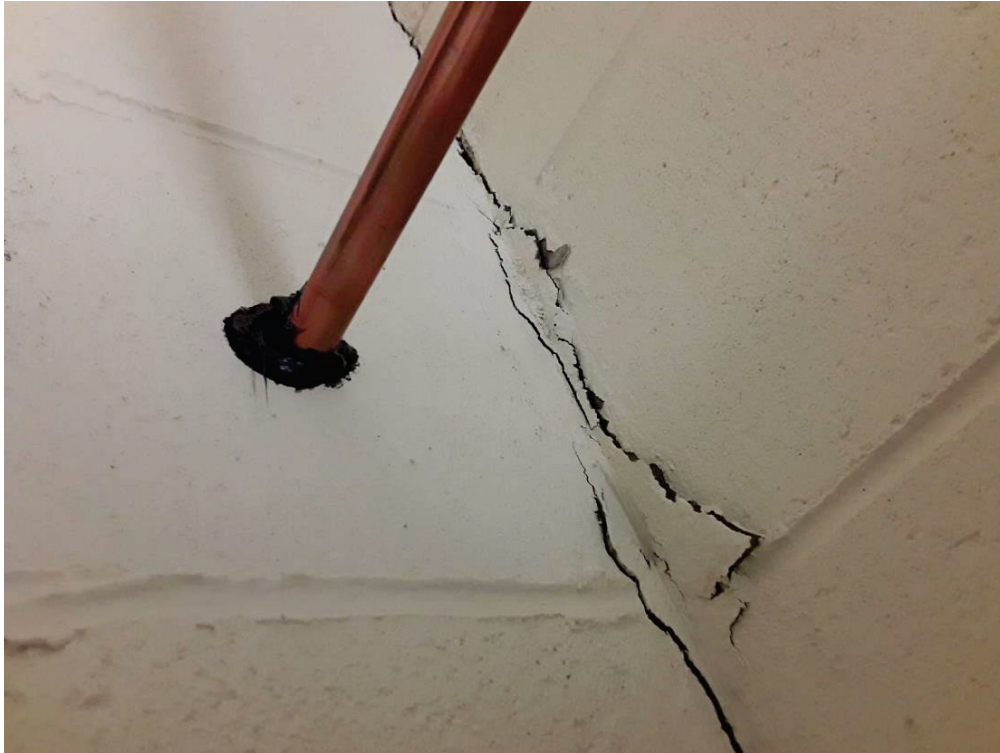
S0003A (None), Firestopping (mastic), Black, C134 Storage (Location #: 7) Wall penetrations
