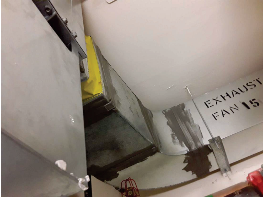
S0001A (None), Duct, Mastic, Grey, C134 Storage (Location #: 7)
